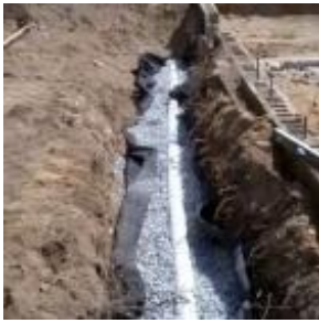
Perimeter Drainage Vancouver
